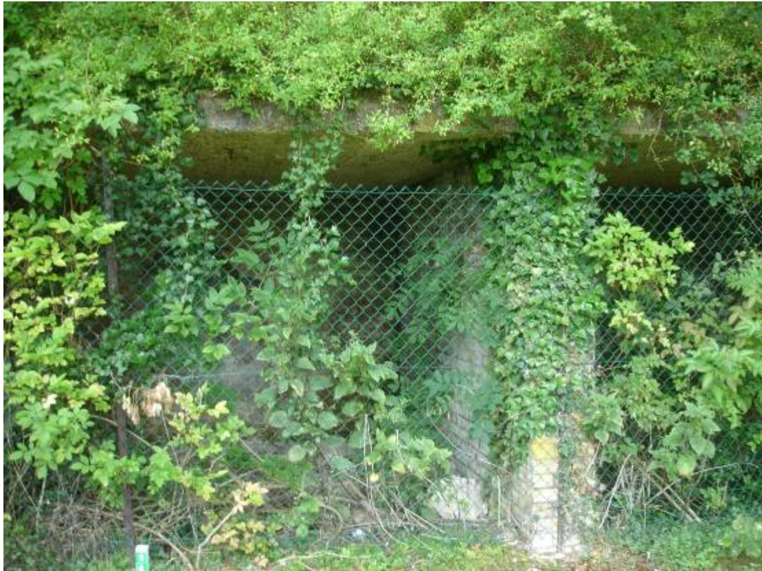
Figure 3: View of concrete shelter containing gaps which may be suitable for roosting bats
