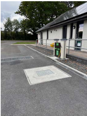
MHSP at Toilet Block B
