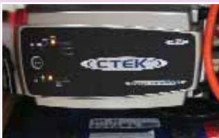
This CTEK charger with maximum charging current of 25A is installed in a motorhome alongside a 180Ah battery
