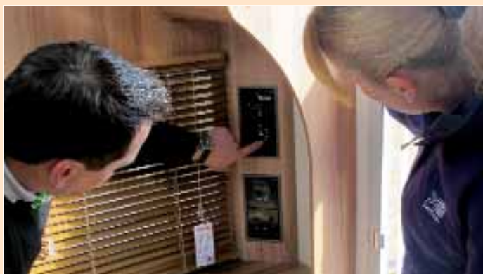
Controls for the Whale space heater are explained and the under-floor device is fired-up
