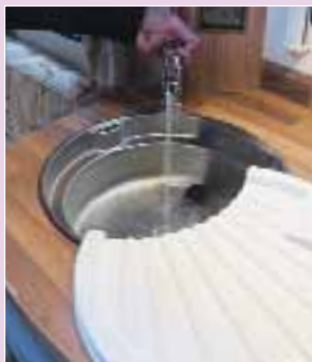
A water supply is connected so that the taps, water heater and shower controls can be checked
