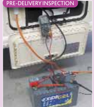
With the 230V and 12V supply systems connected, output from the onboard battery charger is checked
