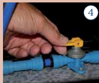
4. Whenever there's a chance of frost, it's essential your water heater has been drained down
